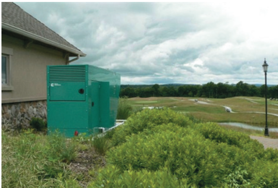
The 100 kW GGHH generator set, installed near the clubhouse, with the course in the distance.
